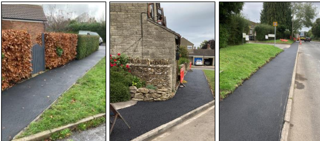
A programme of resurfacing and renewal is underway to improve the condition of the footways.
